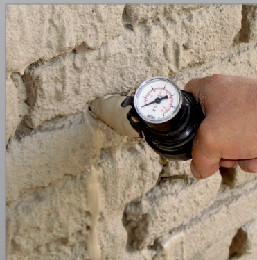
Injection with pressure indication
